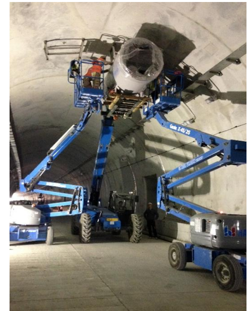
Only five workers were needed - two in each boom and one on the telehandler
